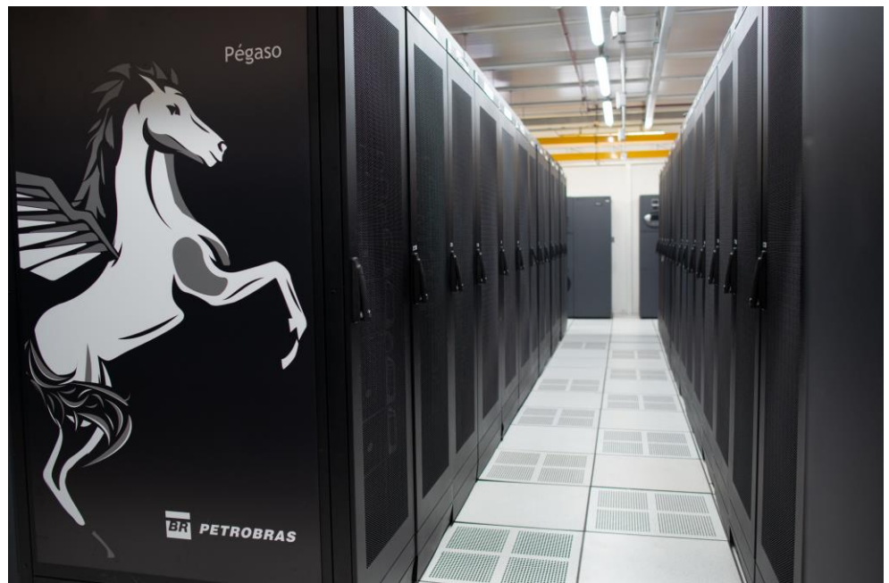
Figure 1 – Pégaso Supercomputer with Supermicro Servers
