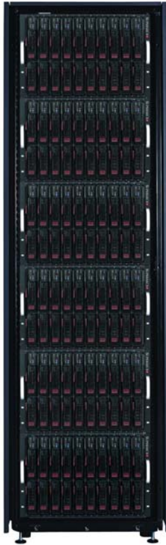
Figure 1-1. Full Rack of Blade Enclosures and Blade Servers
